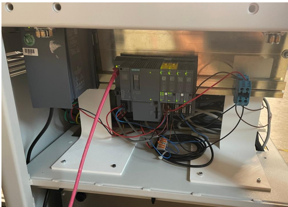
Figure 16: Safety PLC integrated to the pedestal of the Kawada Robot.
